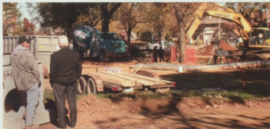
construction corner A contractor from Kissick Construction discusses STA parking lot plans with a worker. The building of the parking lot took a month to complete. photo by emily baker
