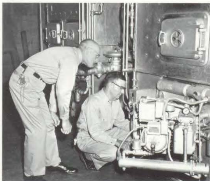
Regulating the furnace in the boiler room is a very important job of Don Barham. George Davenport, head custodian, watches as Mr. Barham checks a small valve.
