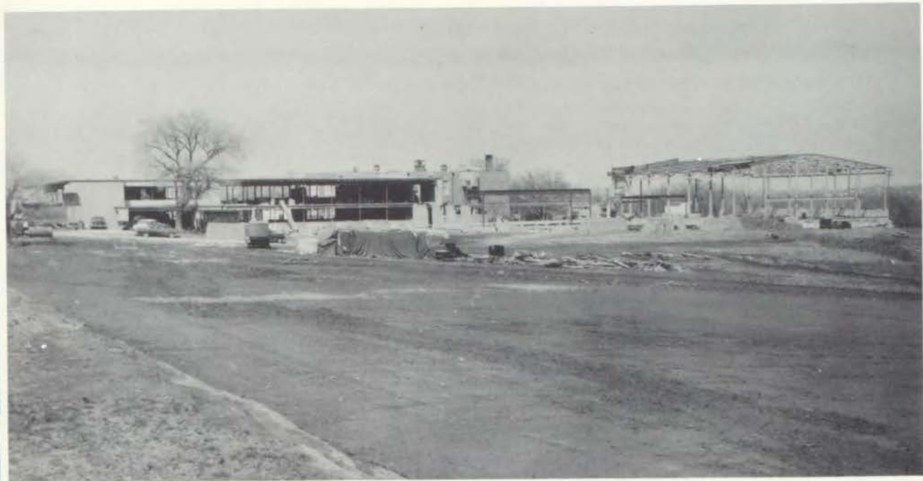
Our new building as it appeared from 24 Highway and Noland during construction stages. The parking area appears in the foreground.
