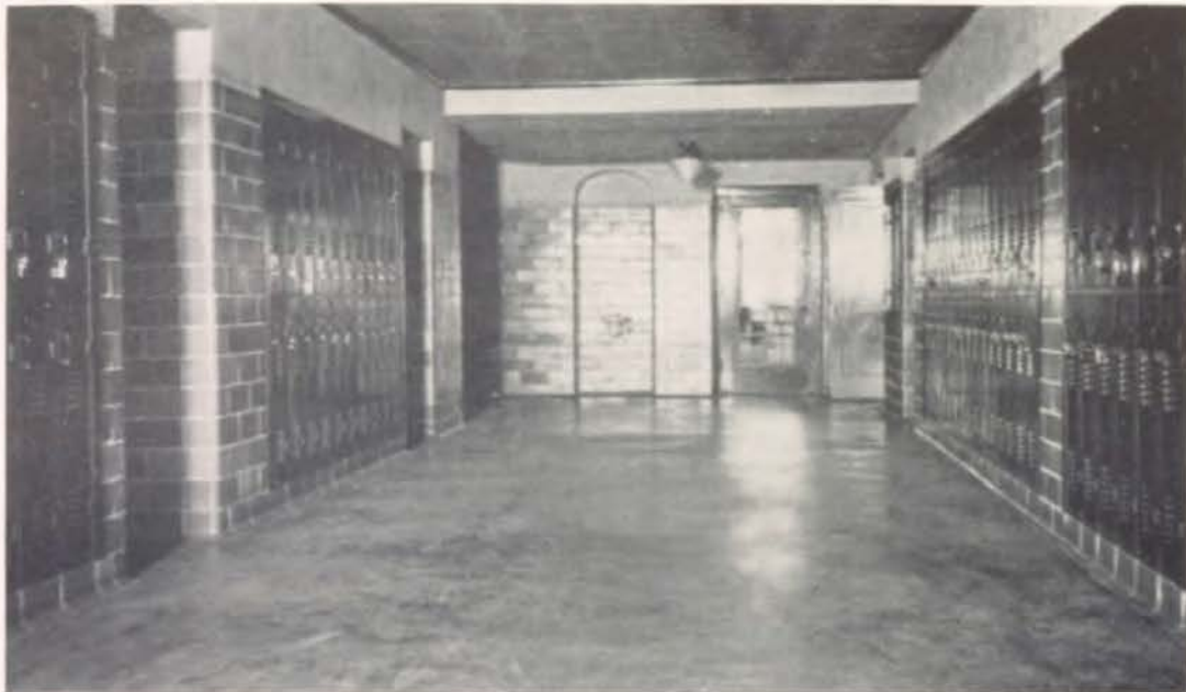
LOOKING NORTH FROM THE SOUTH ENTRANCE ON THE FIRST FLOOR. All the halls of the Annex are lined with lockers.
