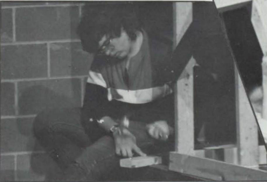
Before attaching the stairs, senior Devin Haynes constructs a landing sturdy enough to support someone's weight.
