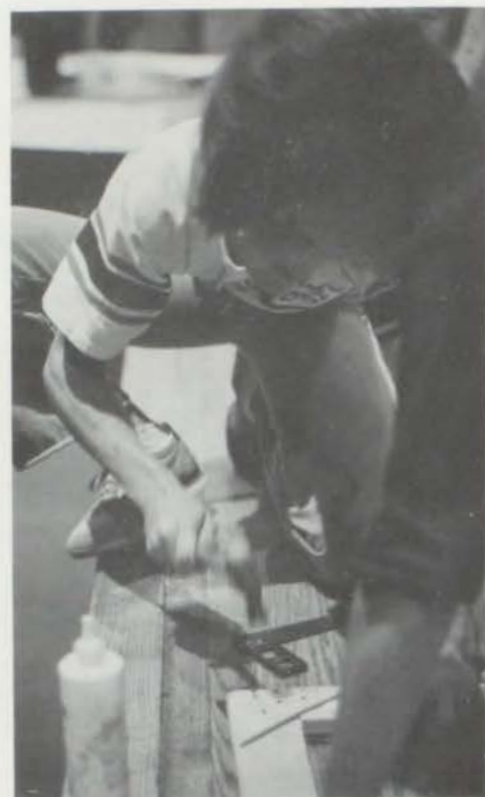
Right: After setting the flats up Gary Sell fits the two walls together as Ken Hearne watches. Below: Flats used for the fall play, "The Desperate Hours," are nailed securely to ensure their strength.
