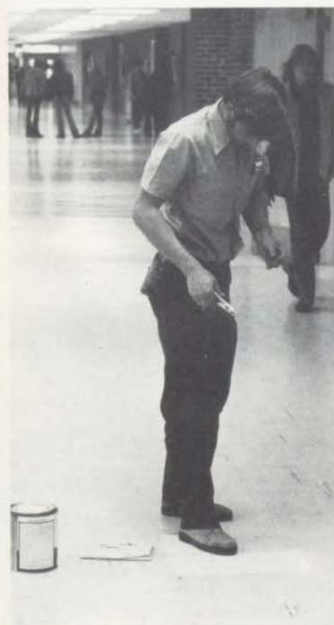
Jack of all trades... Jim Todd retiles a hole in the floor as one of his many custodial duties around school.
