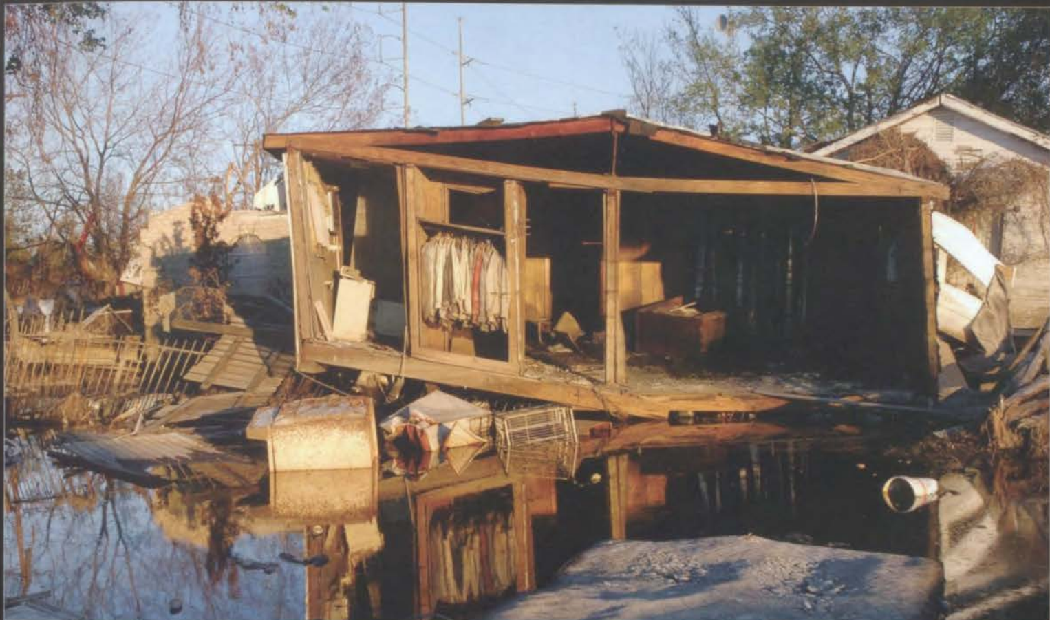
BARELY STANDING Clothes still hang in the closet of one of the hurricane damaged homes in the upper portion of Lower Ninth Ward in New Orleans, Louisiana. The storm inspired Americans to support the states that were victims of the hurricane. PHOTO BY KRT CAMPUS
