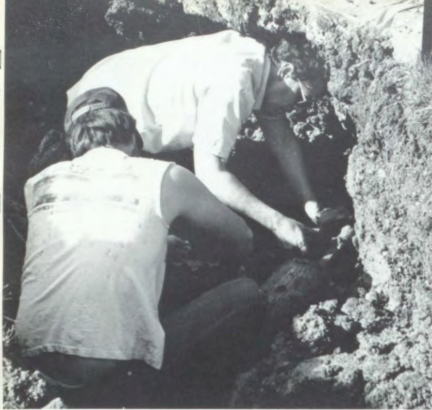
TRYING TO FIX a gasline that had a leak in it, two Kansas Power and Light company employees work to repair the damage (photo by Jeff O'Dell).
