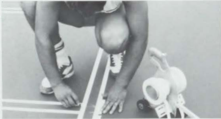
FINISHING TOUCHES ARE added to the resurfaced tennis courts that had developed dangerous three inch cracks (photo by Dina Guarino).
