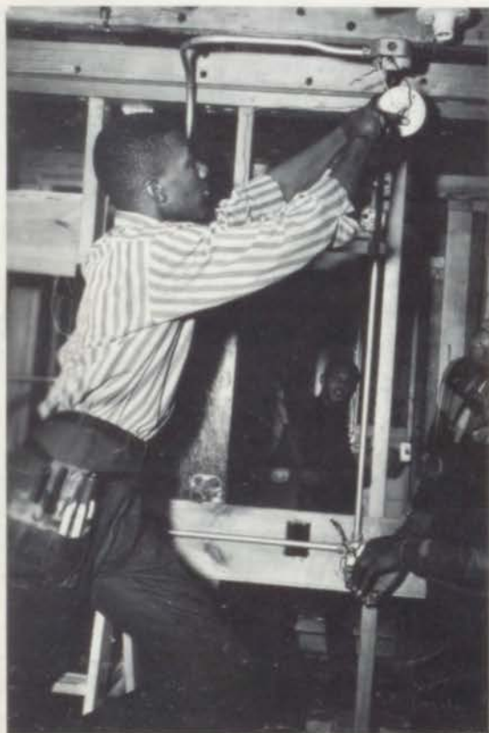
Class in interior wiring-Robert Allen is shown attaching a fixture to an outlet in a room he has wired in conduit. Gene Dudley is looking on. Norman Riley and Ferguson Sanders are looking at the operation from their wiring booth.
