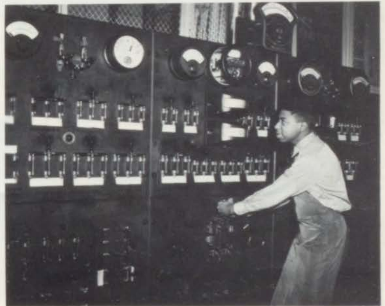
Below: Norman Riley is shown operating a lever on the main switchboard that supplies power to all the machines and work benches in the shop.
