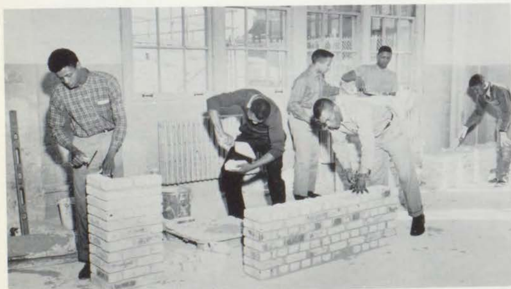
From Left to Right; Clarence Yarbough is working on a 12 X 16 pier, Wardel Griffin and Arthur Jackson are working on an American bond wall, while James Lounce and Ivy Car are working on a 12 X 16 pier, and Jerry Lark is working on a 13' wall.
