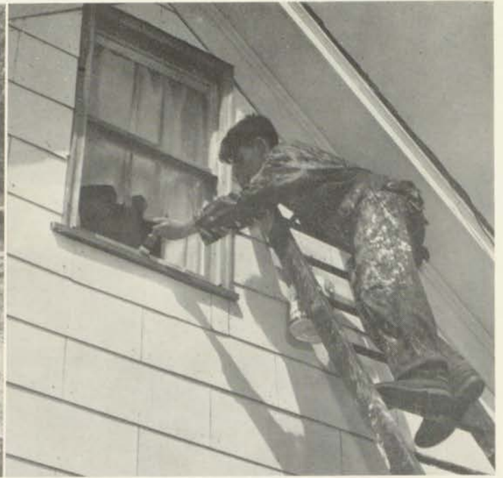
The building receives a new coat as Jack Ballas perches precariously on a ladder.
