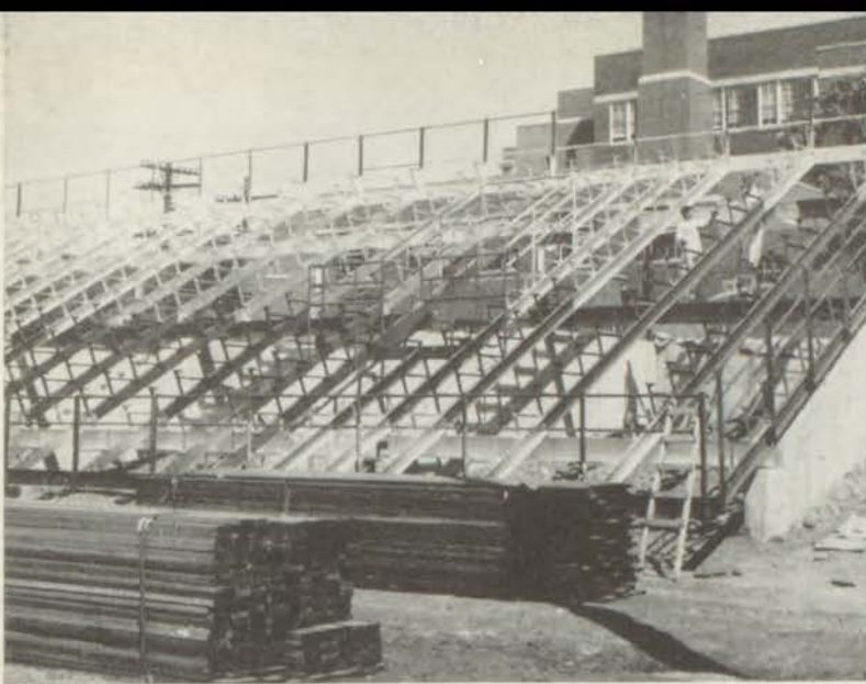
PILES AND PILES OF WOOD were heaped in front of the metal skeletons of the bleachers as the stadium was erected.
