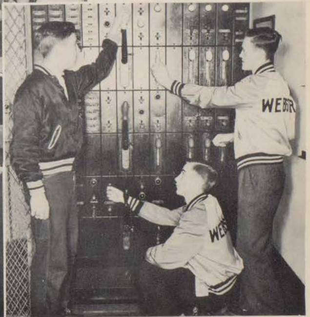
Below: Bob Stuckey, left, and Bert Larkin, captain, kneeling, are consulting with a fellow stagecrew member, David Fricke, on the intricacies of the stage switchboard.
