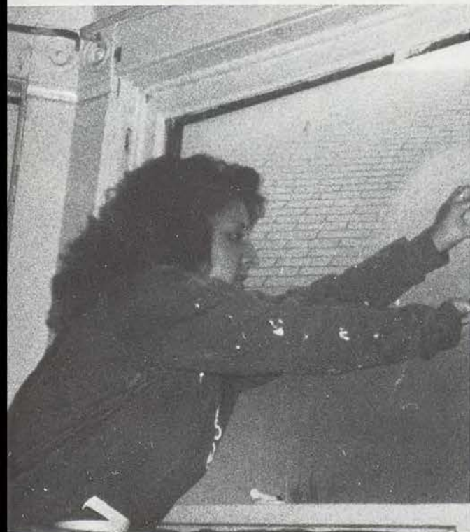
Helping a family that couldn't afford to better insulate their home, President Lisa Shiflet (12) places caulking donated by the Kansas City Chiefs in a window. Photo by Susan Wolf
