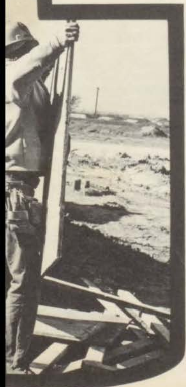
They were still working on the Civic Center. Now, however, the workmen had started to put up walls. Slowly but surely the building took shape.
